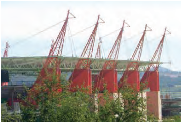
Mbombela Stadium, Nelspruit South Africa Client - Mbombela Local Municipality Structural Engineer - Mott MacDonald
